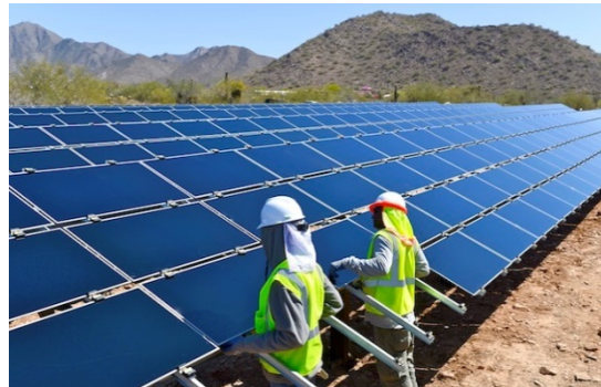
Ground mounted solar PV system.
