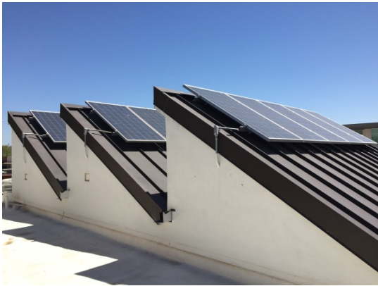
Roof top building integrated system.
