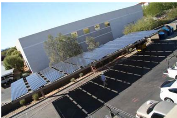
Solar PV carport structure.
