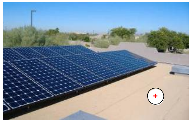
Solar panels on flat roof with parapets.
