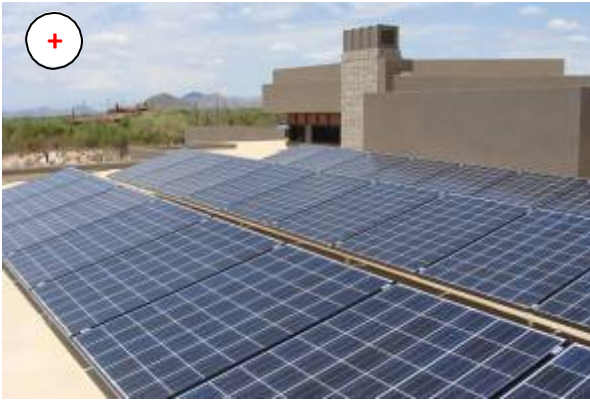
Solar panels on flat roof without parapets.
